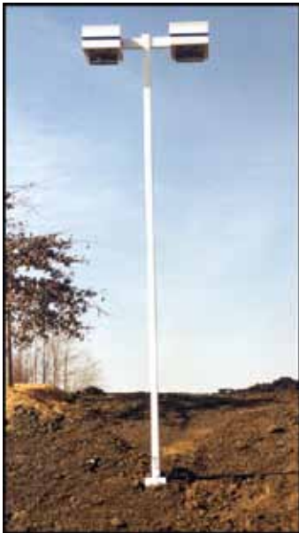
Installed Light Standard Figure 10-2
